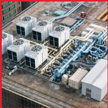
Air Handling Units
